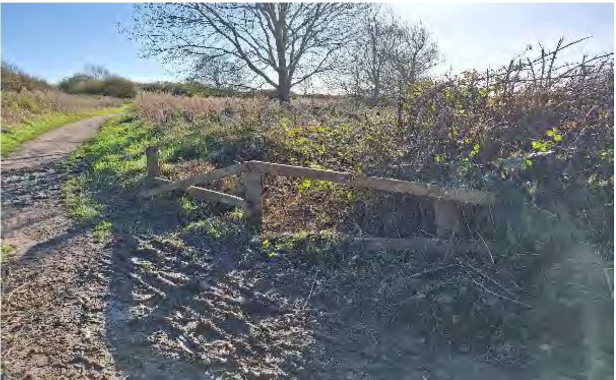
Photo of fence requiring repair to assist with locating – on red route adjacent to a natural brook.
