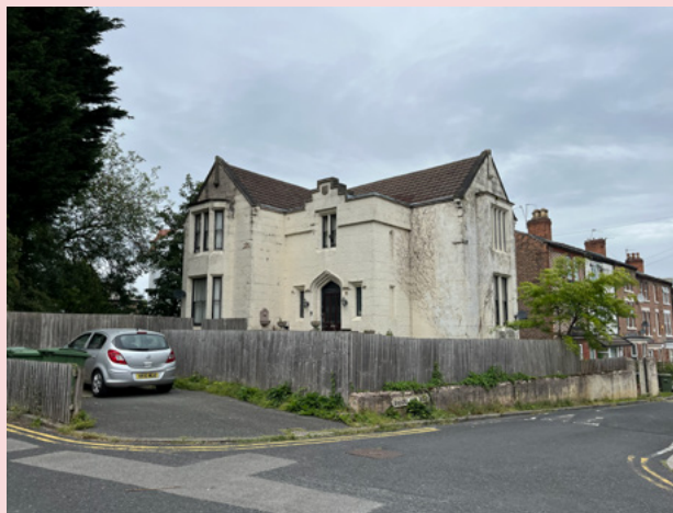
6.2.4 Poor condition to historic building, including inappropriate paintwork
