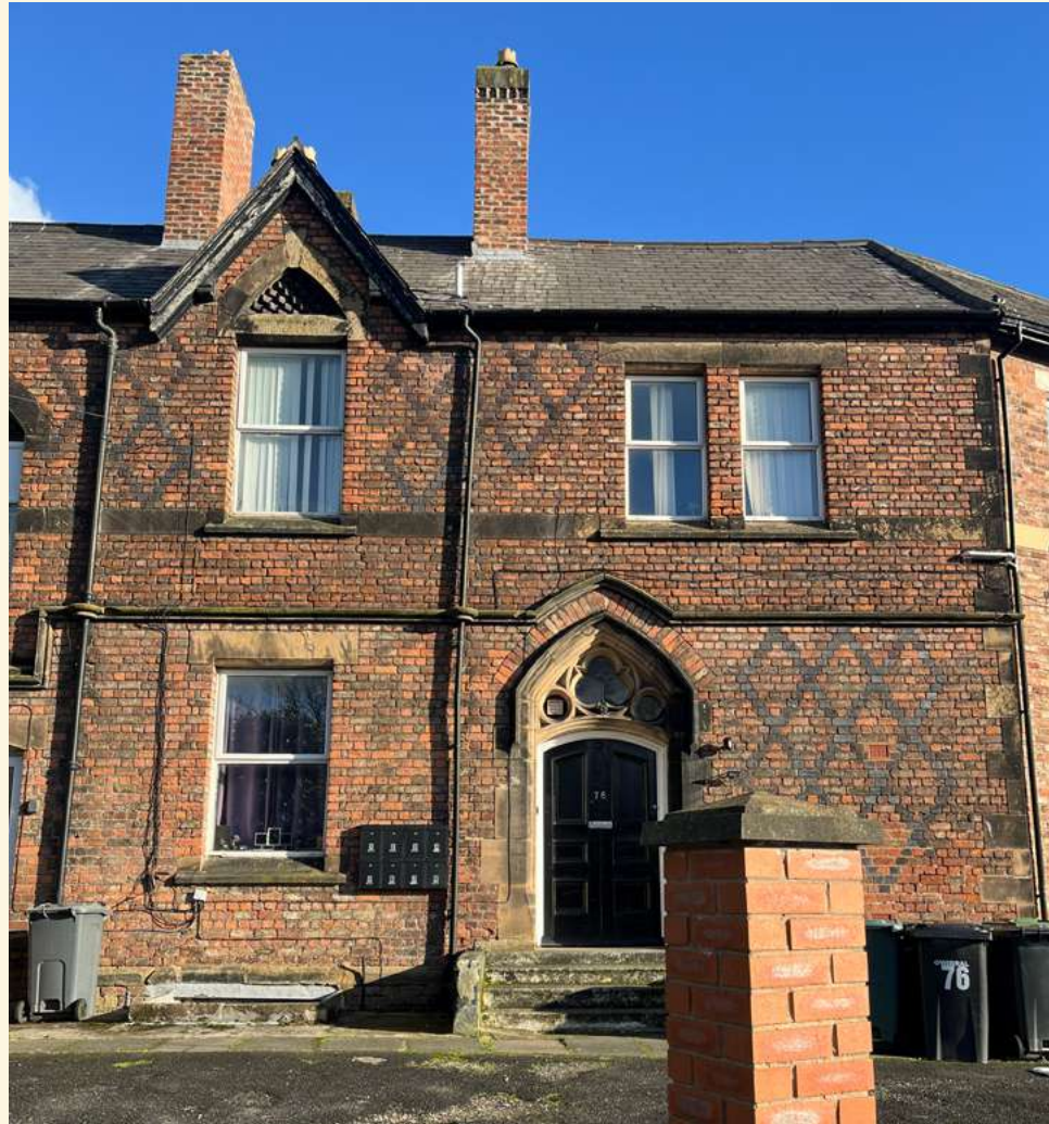
6.2.14 Villa in need of repointing
