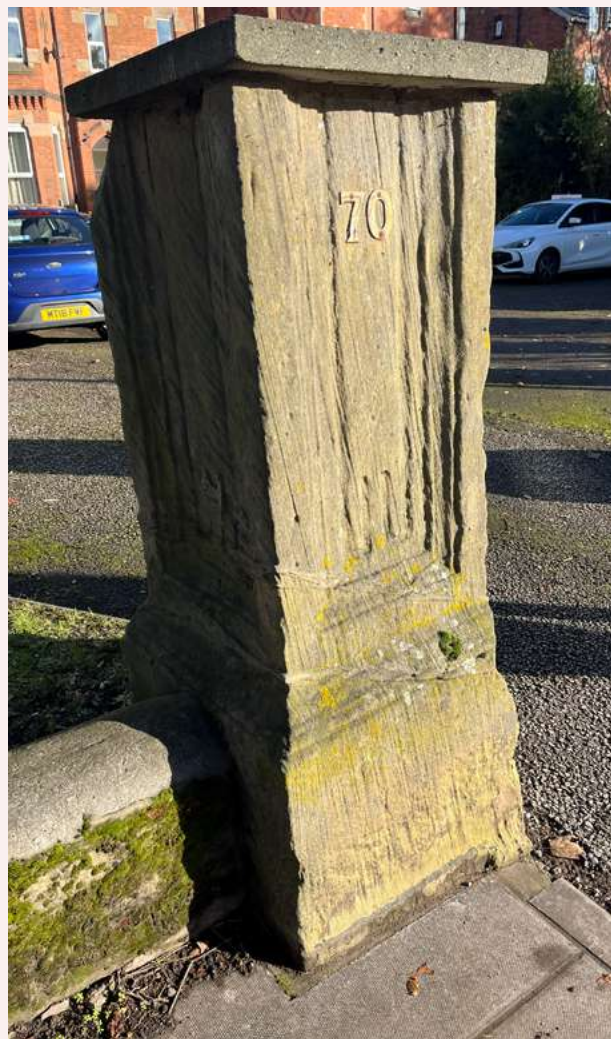
6.2.12 Damage to historic gate pier
