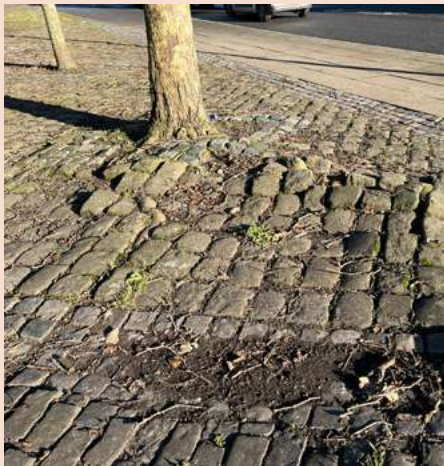
6.2.15 Cracking and damage to paving by roots
