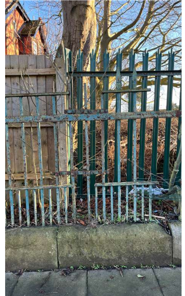
4.12.43 Poor quality gates and fencing behind historic examples at Staveley
