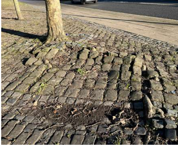
4.3.24 Paving disrupted by concrete blocking
