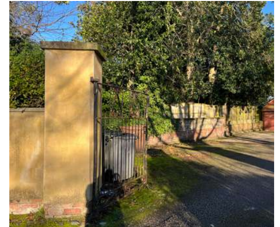
4.3.30 Poor quality rendered pier
