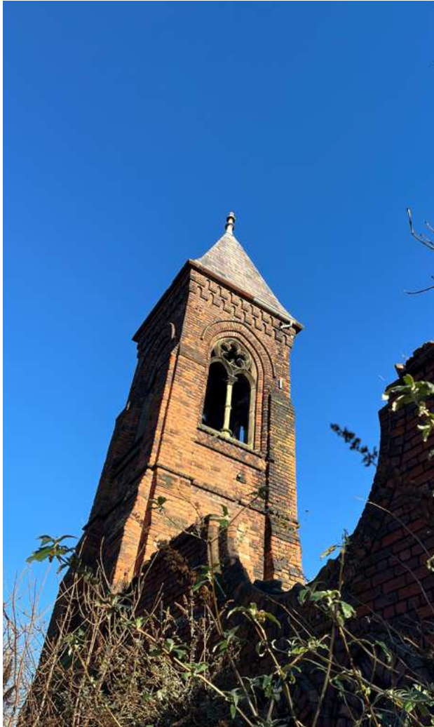
5.1.10 Former Apostolic Church in derelict state
