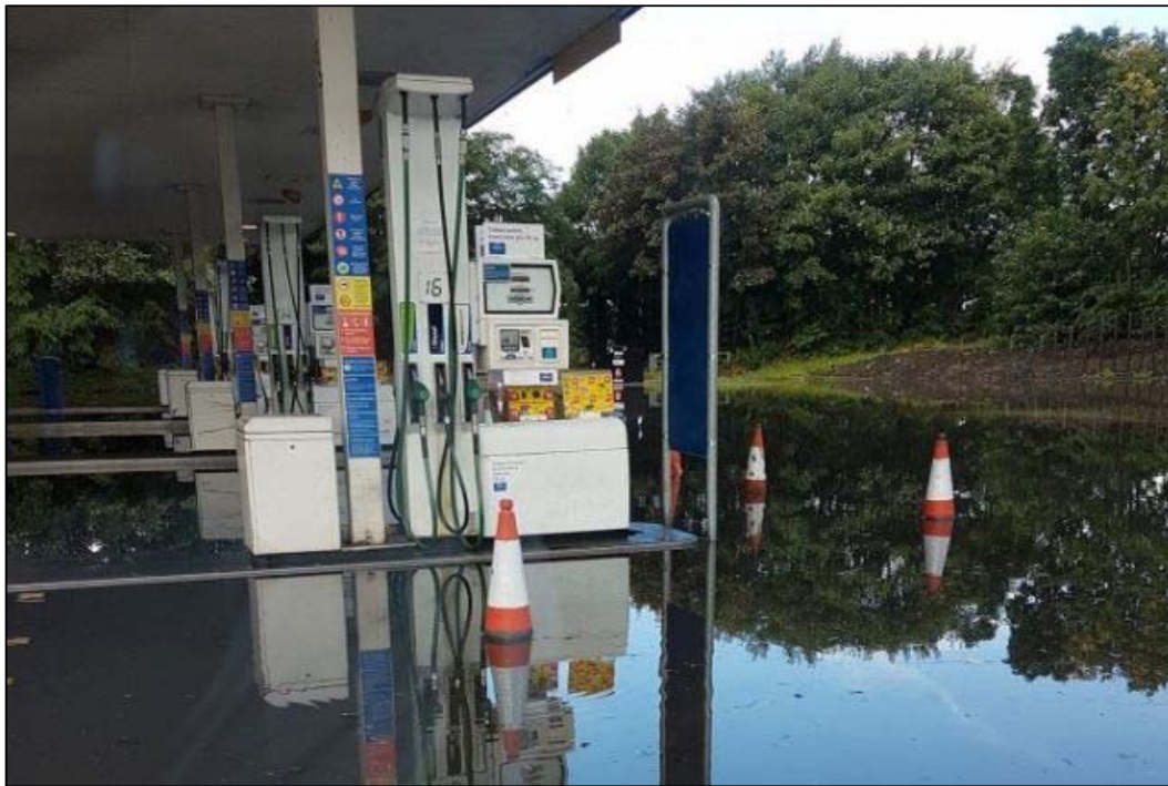
Figure 6: Surface Water flooding at Tesco Petrol Station, 23 rd July 2017
