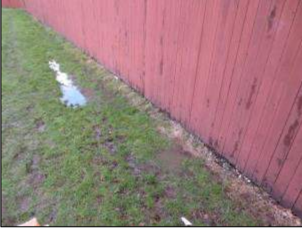
Photograph 5-6 Surface Water behind Brookdale Close (1/3/16)
