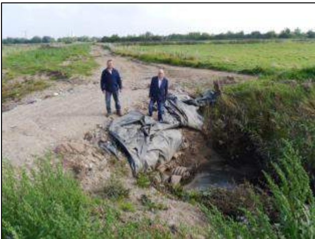
Photograph 5-26 Arrowe Brook, UU structure (post-event photograph)
