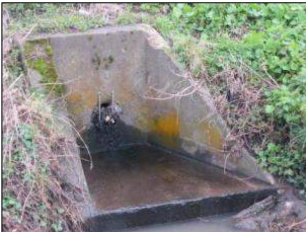
Photograph 5-23 Blocked Surface Water Outfall (2/3/16)
