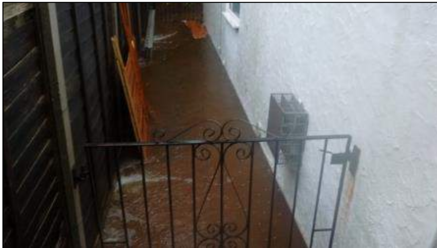
Photograph 5-8 Flooding at the back of Joan Avenue (2/9/15)
