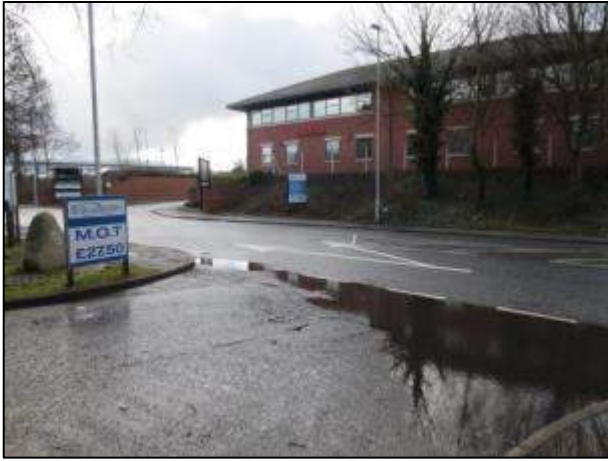
Photograph 5-30 Low spot on the Prenton Way (3/5/15)
