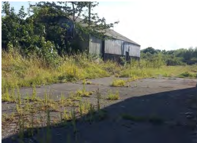
Sheds and glasshouses are in a dilapidated condition
